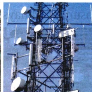
Under the pilot project titled SMARTSEL, the govt has allocated RM3m to develop 5G infrastructure at the state's secretariat building
